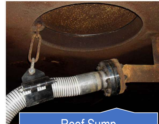
Roof Sump Connection
