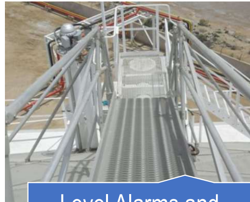
Level Alarms and Penetrations
