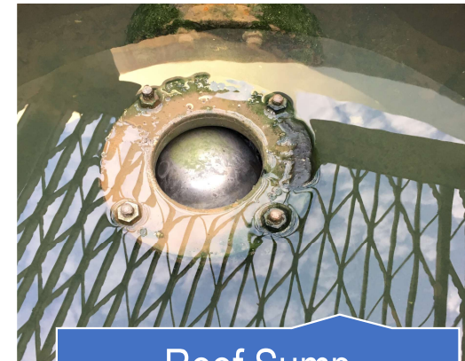
Roof Sump Drain Valves
